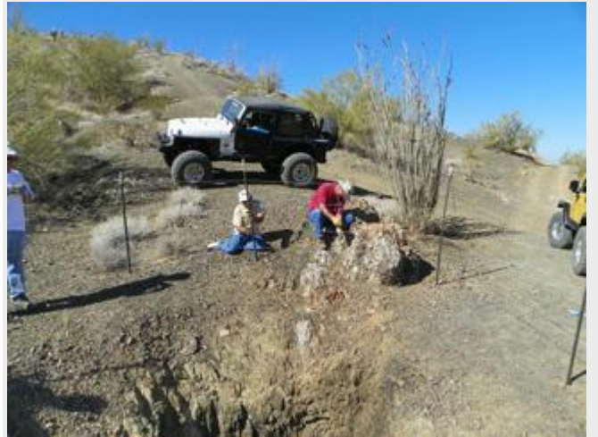
Havasu 4 Wheelers work Thursday to fence open vertical mine shafts in desert areas near Lake Havasu City during an extended effort and partnership with Bureau of Land Management. Submitted photo
